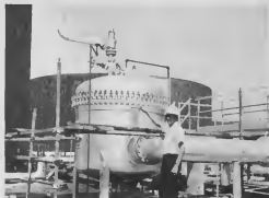
Camilo Daal of Mech-Engineering shows one of 219 special filter cartridges contained in this milli-pore jet fuel filter unit. This new filter system helps assure maximum product cleanliness.
